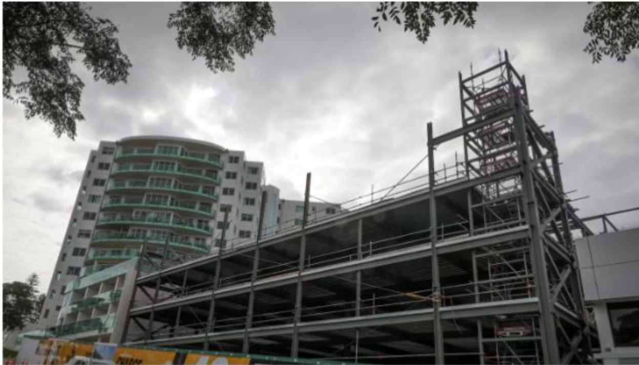
Harington St Transport Hub, pictured after work was abandoned on the project. Photo / Andrew Warner
